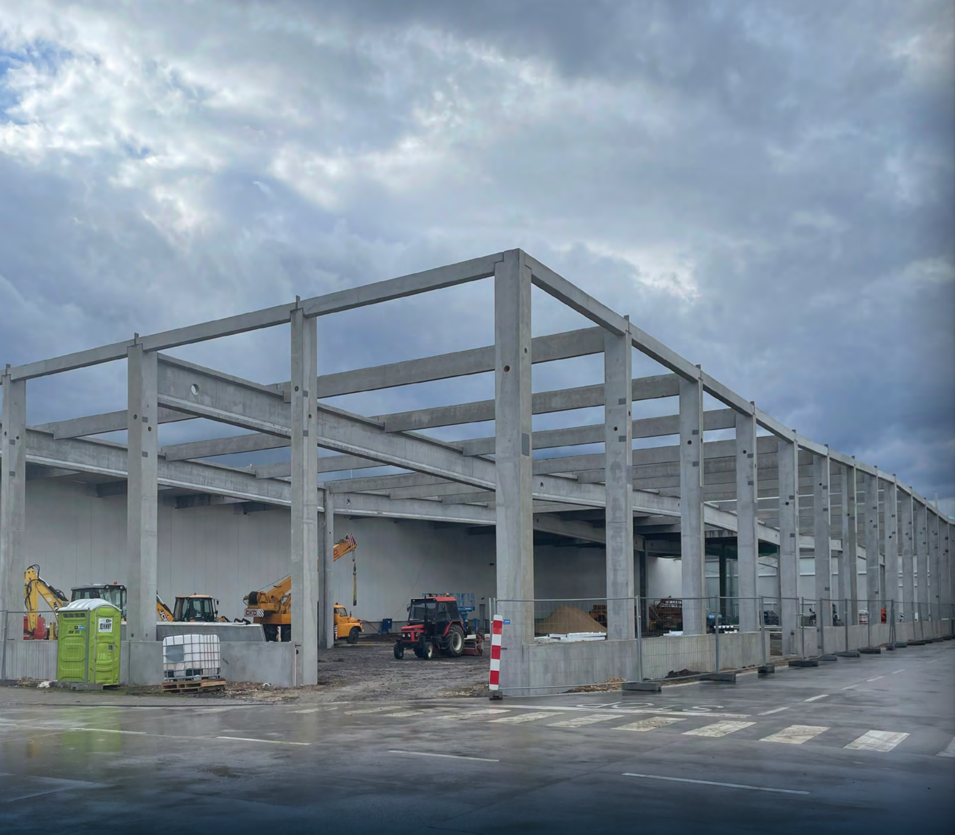
Construction of the skeleton of the warehouse hall in the Géňa Industrial Park in Levice in March 2023.
